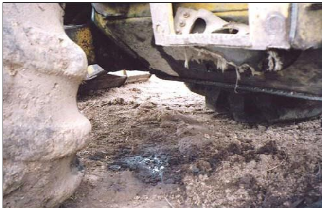
Oil leaking from machinery.
